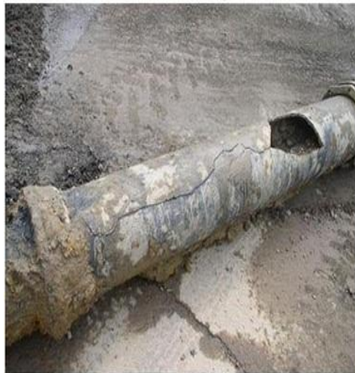
Fig. 1: Cast iron pipe broken from water hammer
